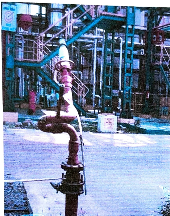
Annexure III – Picture of Fire Fighting:
